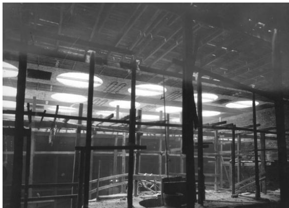
Radiant ceiling heating coils by Crittall, 1935. Photo: Alvar Aalto Museum.
